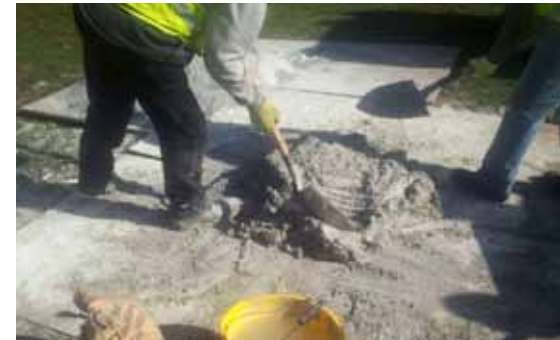
Small quantities of mortar can be mixed by hand which was the traditional method. Note the steam rising
