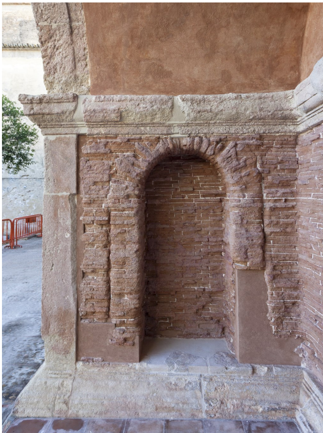
Volume reintegration in the most damaged areas of the brick fabric with lime putty mortar.
