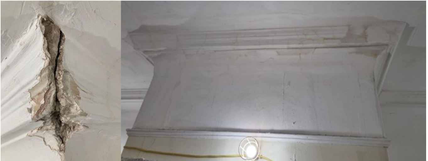
Left: Damage to junction of cornice over fireplace. Right: Patch repairs to plasterwork of chimneybreast.
