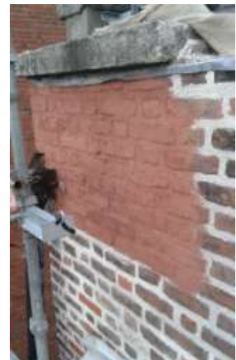
Raddle coat being applied to the façade of Tailors’ Hall. James Kelly, Architect & Old Stone, Masonry Specialists (Ref. Nicki Matthews, C.O.)
