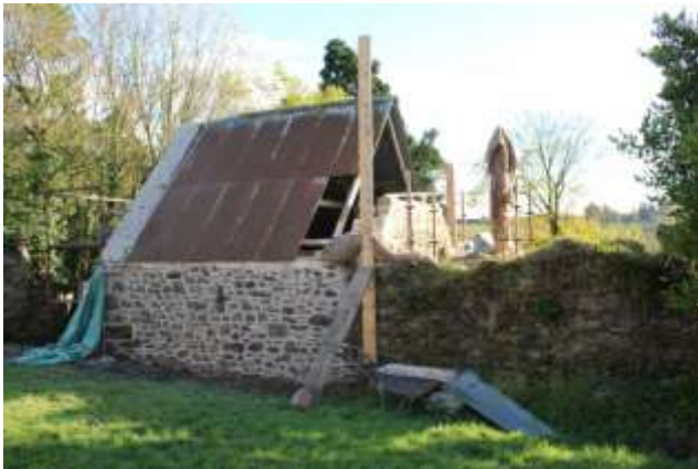
Gable with missing top-section
